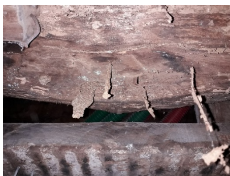
Figure 1. Cocoons on one of the main beams of the 1st floor structure (ceiling of the Non-Teaching Staff Room)
