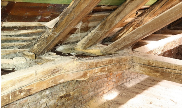
Figure 2 a)-c). The brittle bending failure of the grid beam is attributed to the inadequate positioning of the rafter at the end of the tie beam, resulting in eccentricity that causes upward spur rotation. The tie beam further bends due to insufficient support beneath the queen post (upper right). Right: the current configuration with a single wall plate (left), and the proposed configuration with two wall plates and iron braces (right).
