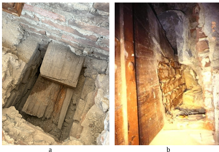
Figure 24. (a) Ventilated cavity in the masonry; (b) Inverted C-shaped stone above the rafter and the fungal decay on the tie beam end
