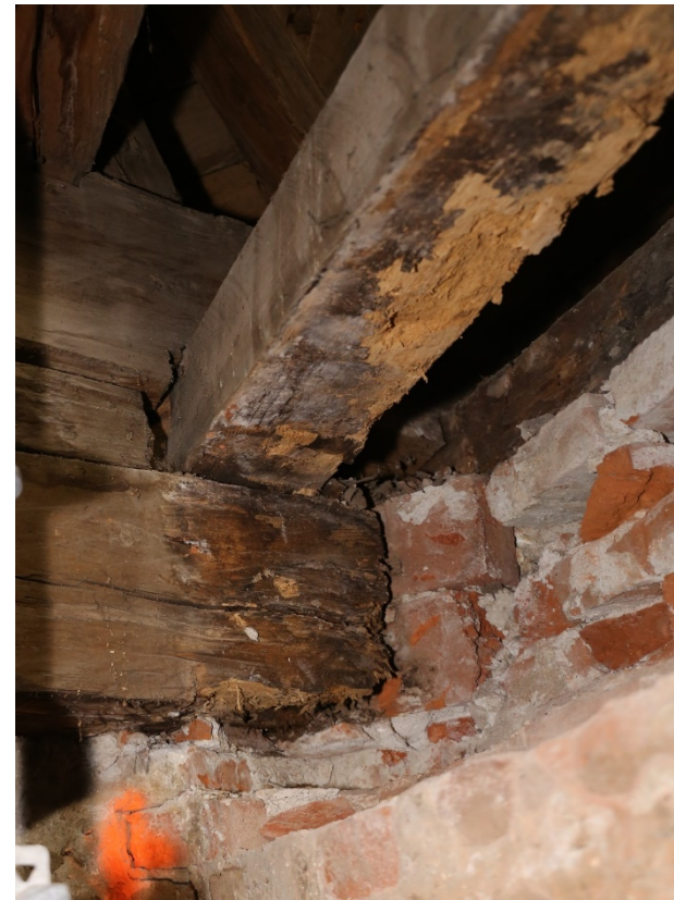
Figure 6. Severe damage to the support of the truss of the central nave of the Zagreb Cathedral (1888), with still ongoing decay activity.
