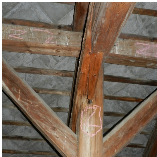
Figure 3. Loose connection of the strut and queen post
