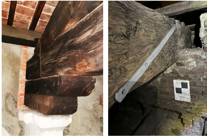
Figure 23. Examples of enlarged masonry pockets at the truss ends
