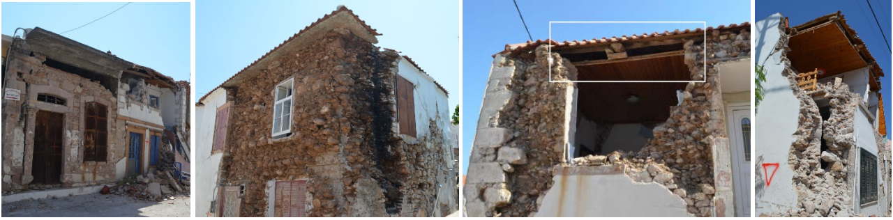
Figure 1: Vrisa village in Mytilini, Greece. 2017 earthquake. Severe damage and partial collapses were observed in masonry buildings reinforced with concrete slabs and concrete tie-beams at roof level, and in masonry buildings without timber lacing [6].
