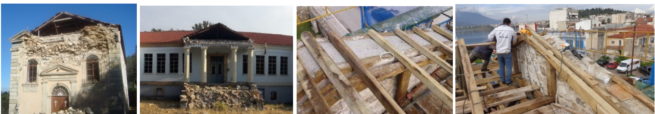
Figure 6: a) Kefallonia (2014), b) Mytilini (2017). Typical gable collapses caused by earthquakes. Bailos House in Chalkis. c), d) Timber lacings anchored with steel rods to the masonry are used to connect the gable to the roof inclined diaphragm, through the purlins that are screwed onto the timber tie beams [11].
